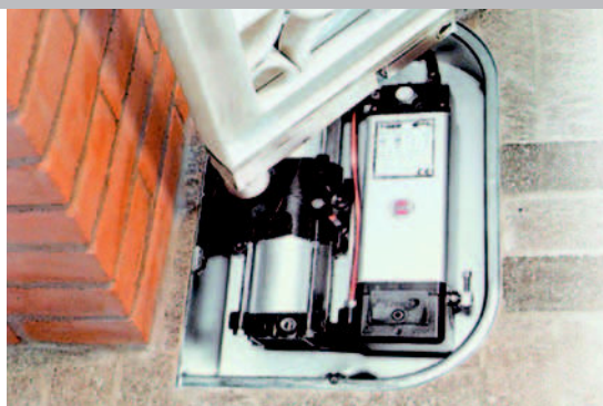
Equipment in working condition
